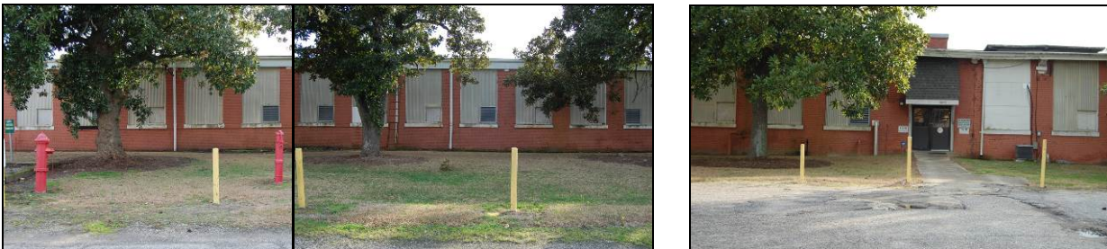
Figure 83. Eastern section of north front elevation; note altered window bays and, at right, entry
