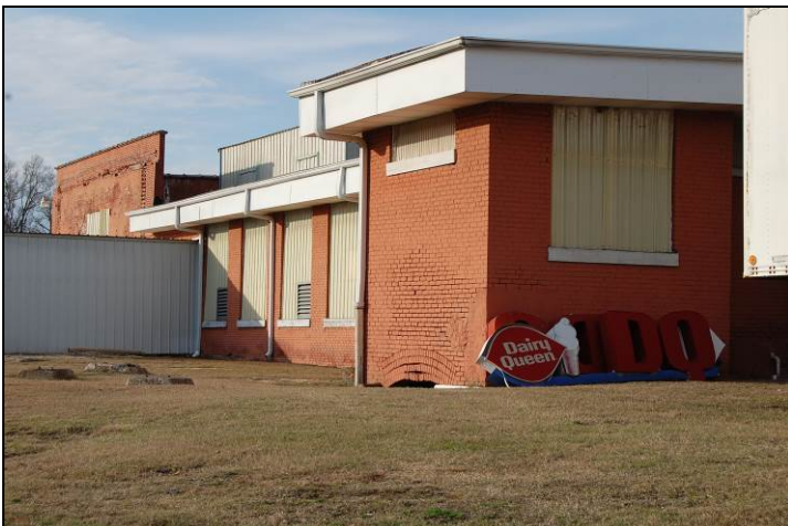
Figure 90. Detail of eastern portion of south elevation; ghost marks of former powerhouse visible at parapet wall at left
