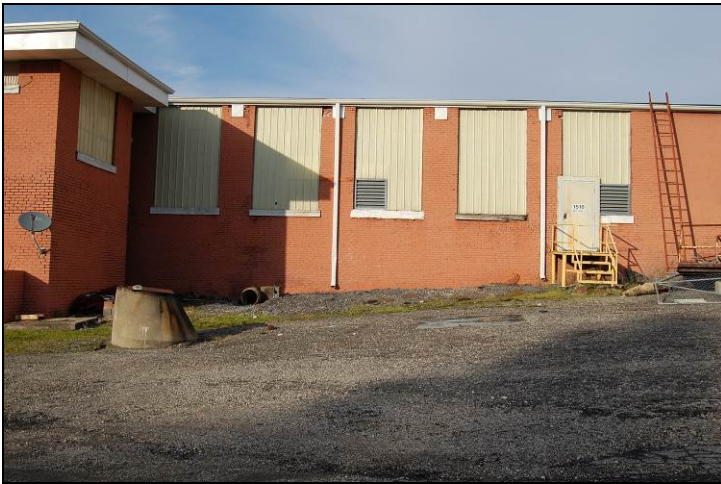
Figure 89. Detail of western portion of south elevation with windows covered by fiberglass panels and, at right, red-painted concrete-block infill
