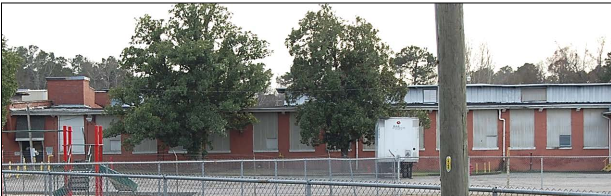
Figure 84. Western section of north front elevation with entry at far left; note altered bays and sheet-metal-clad clerestory
