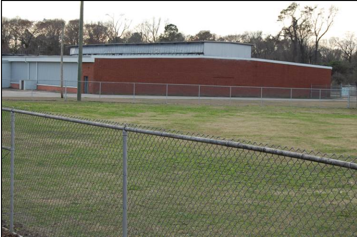
Figure 85. East and north-facing elevations of 1927 knitting room; note post-1957 covering of window bays and clerestory with sheet metal and brick veneer
