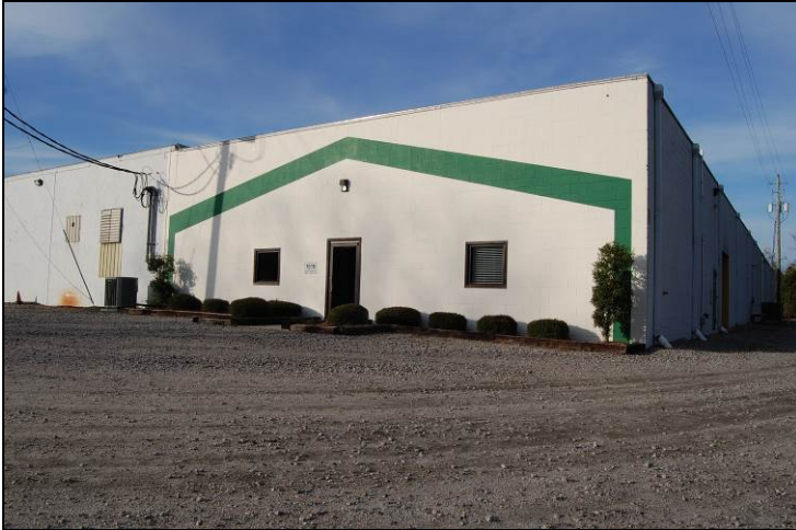
Figure 91. South rear and east side elevations of c.1957-1965 concrete-block addition at mill's southeast corner
