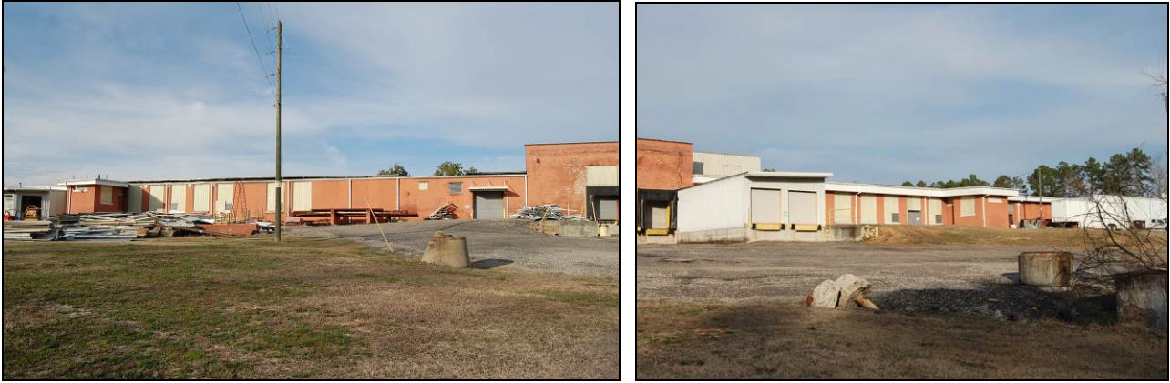
Figure 88. South rear elevation of original mill building; windows enclosed by brick, concrete block, and fiberglass panels
